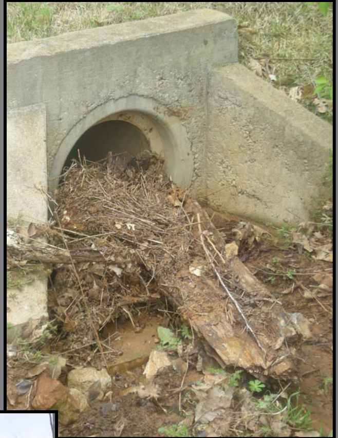
A drain was overwhelmed and plugged
